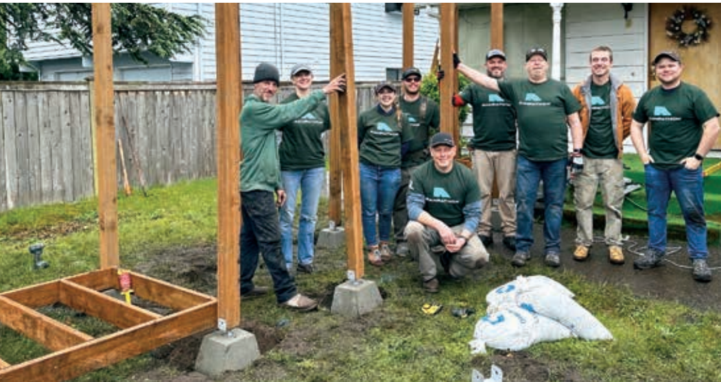
Struggling to climb three steep, concrete steps leading into her home, an 88-year-old Seattle resident applied to Rampathon. Ashworth Homes built a ramp that the recipient claimed to be “an incredible gift to our community!”
