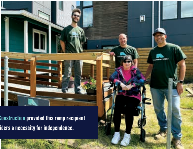
CRD Design Build constructed a ramp for a resident who lives on fixed income in Des Moines.
