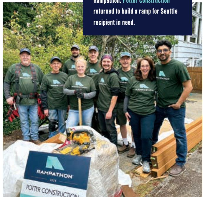
Chermak Construction Inc. helped an elderly couple in Lynnwood gain increased independence through this ramp build.
